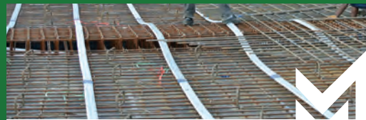
SLAB & SPIRAL DUCT
